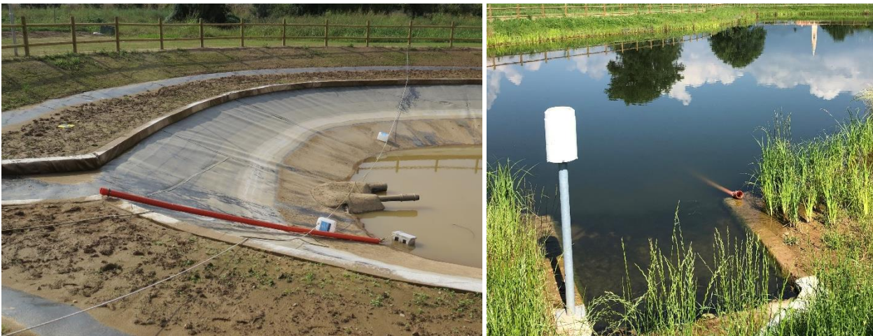
Figure 4.12. The perforated PVC pipe installed on bank of the basin that host the pressure transducer in order to measure the water level.
