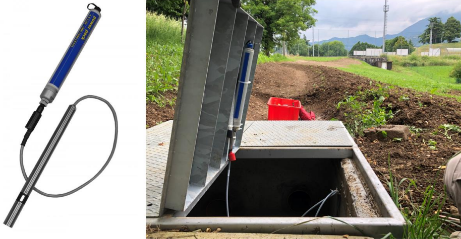
Figure 4.7. The pressure transducer SEBA Dipper-PT used to monitor the flow head over the weir crest (on the left), and a picture of its installation in the Intervention 2 of Action C4 (Grumo hill, Santorso).
